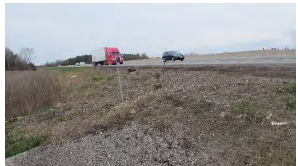
Culvert C474 South – Embankment erosion
