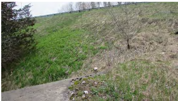
Culvert C473 North – Embankment erosion
