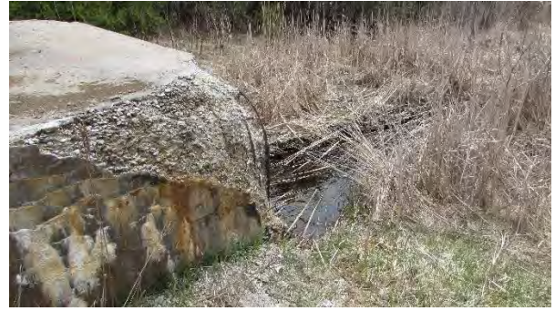
Culvert C473 South – Exposed Rebar
