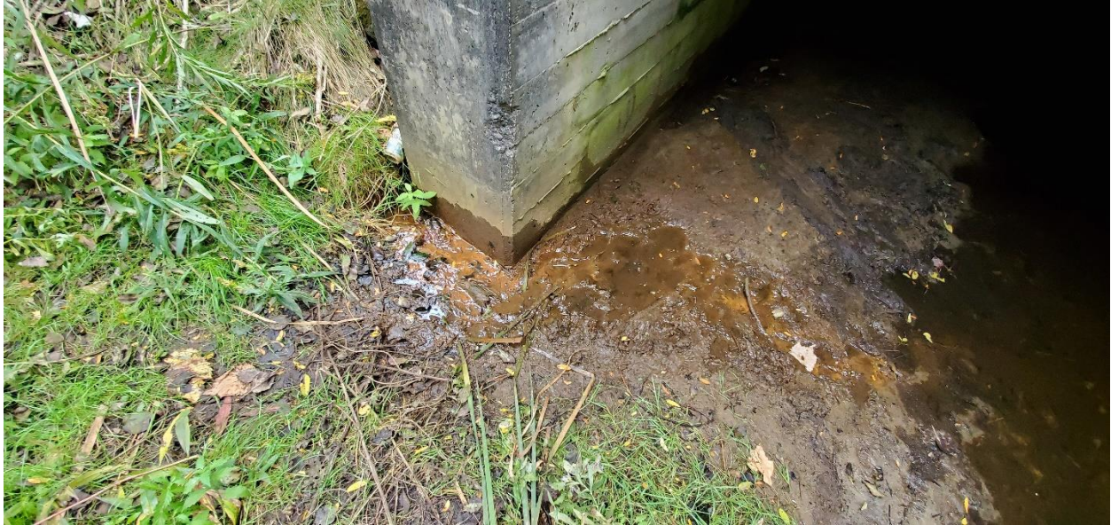
PHOTOGRAPH 15: IRON STAINING OBSERVED AT CULVERT 21-473C, FACING SOUTH
