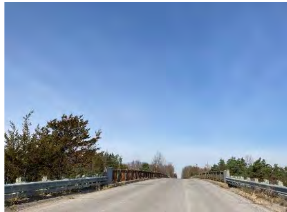
Image 23: View of Lake Road Underpass looking north, note metal post and panel railings
